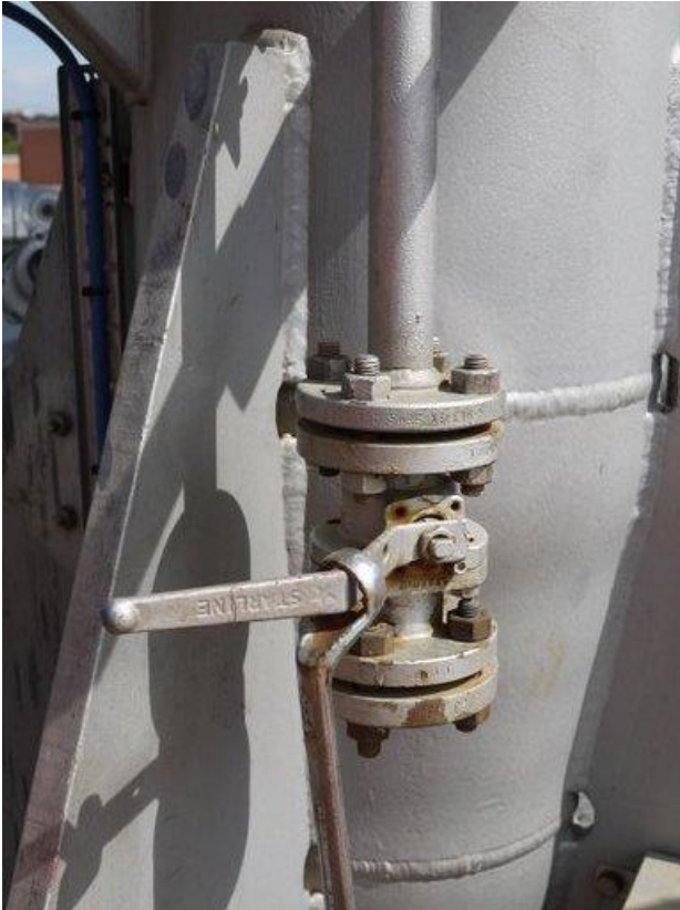
Valve not labelled. Action raised to address
