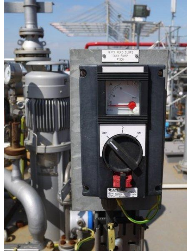
Pump start/stop. Design and layout consistent with others on site. Well located. No issues
